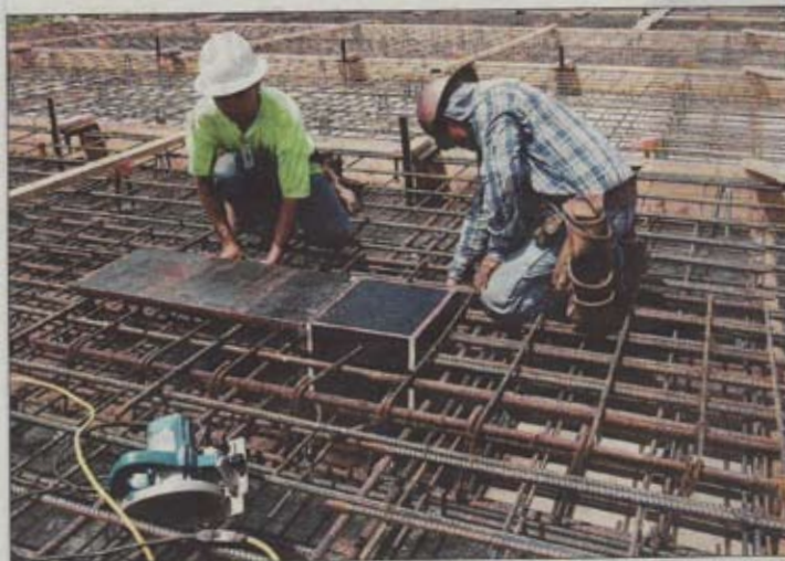
Christian Romero, left, and Jesus Medrano, both of West Palm Beach, use wire ties to reinforce the rebar for the exterior wall of the gymnasium under construction at Hillel Day School of Boca Raton. Staff photo/Kimberly D'Mare
